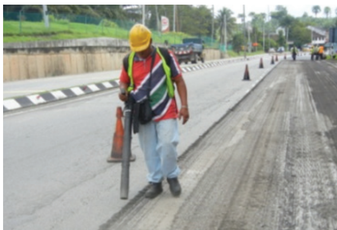
Compressed air blower
