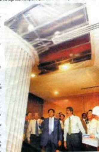
Works Minister Datuk Seri S. Suresh Velu and PWU officers inspecting a defect in the ceiling at Parliament House recently.
