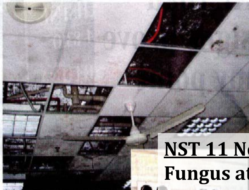
Patches of fungus infection detected at the ceiling of the women's visitor centre at Sultan Ismail Hospital in Johor Baru. (Inset) The hospital's canteen walls are also affected by fungus.
