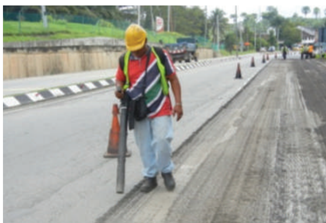
Compressed air blower
