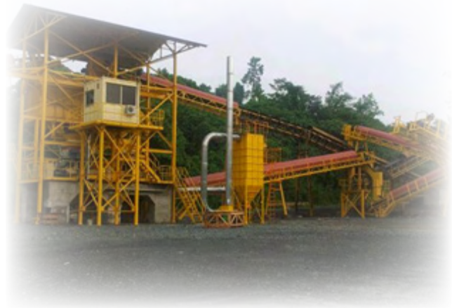
Tertiary dan Quarternary Crusher
