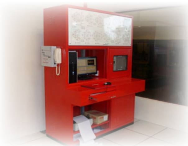
Control Panel Fire Alarm System
